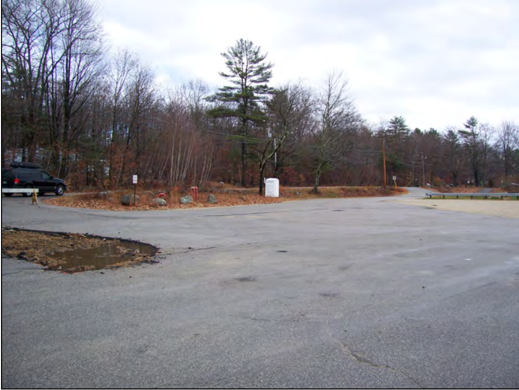
Civil Photo 9: Upper lot, uncurbed landscaped island at left side, looking northeast.
