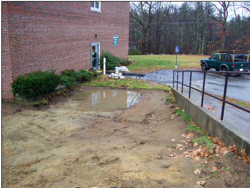
Civil Photo 16: Existing drop inlet and non-ADA compliant handrail.
